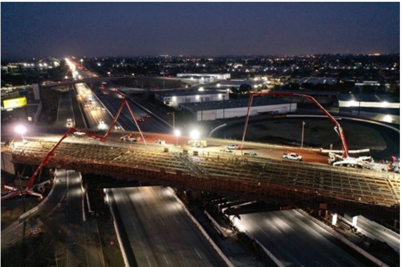
Bolsa OC deck Pour – Crews completed the concrete deck placement for the first phase of the Bolsa Ave. overcrossing bridge reconstruction in the City of Westminster in December 2020. Phase one construction on this bridge is nearing completion and phase two construction for the second half of the bridge is planned to start this Summer 2021.
